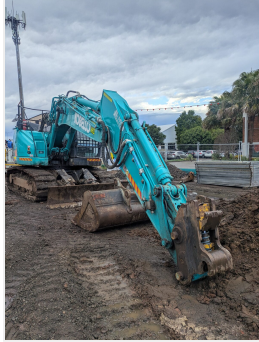
Front Left Corner
